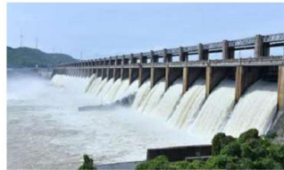
All hands on deck: The engineering emergency evolved into one of the biggest dam rehabilitation exercises in the nation. SRIDHAR KAVALI
